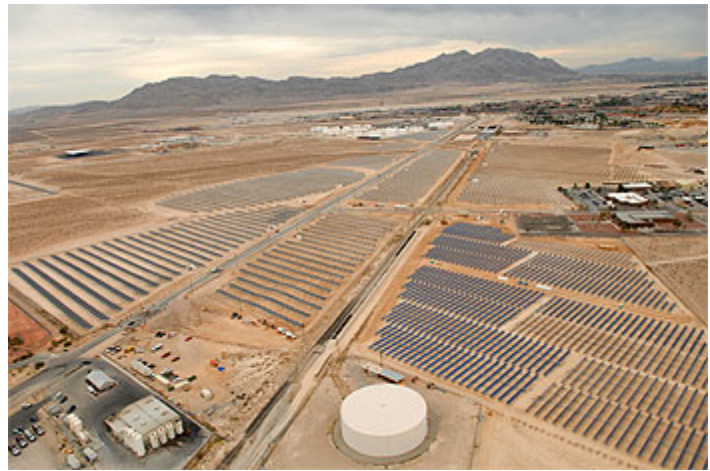
The solar field at Nellis Air Force Base is comprised of more than 72,000 photovoltaic panels. The array is expected to produce more than 25 percent of the base's electricity.
